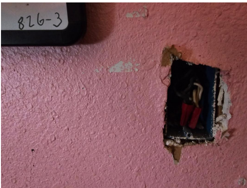
826-3 (Main House) Drywall/Joint Compound Typical Interior Walls/Ceilings
